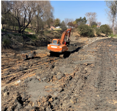
In places, the silt that had to be removed was up to 1.8 metres deep.
