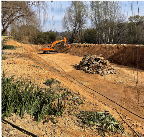
The big guns had to be called in to reinforce the walls.
